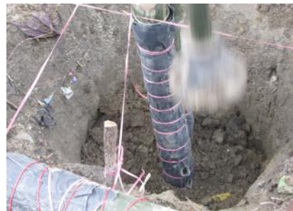
Tampering debris in foundation
